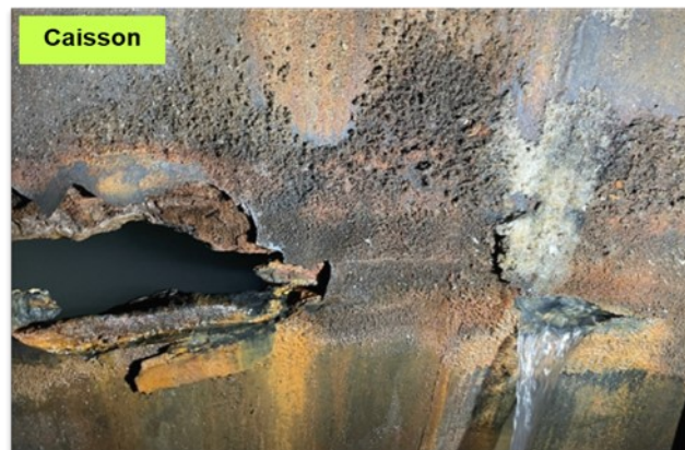
Figure 6. Corrosion failure of caisson wall.
